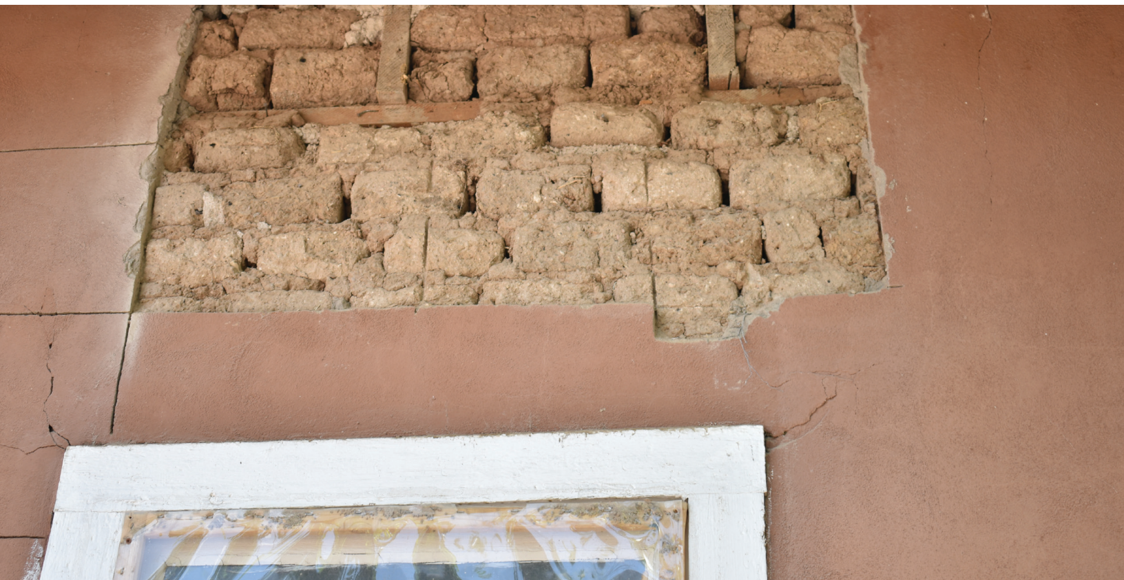
Partially removed stucco and the adobe beneath, The Pino House, photo by Ramon Dorado
