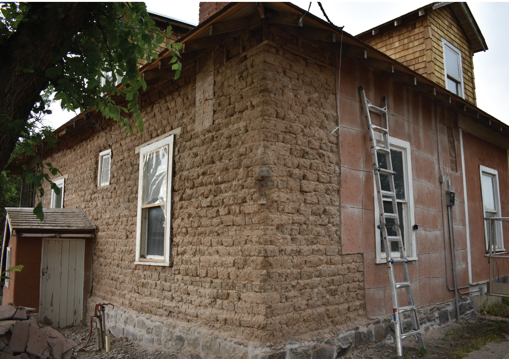
Removal of stucco wall cap in progress at El Zaguán, photo by Ramon Dorado
