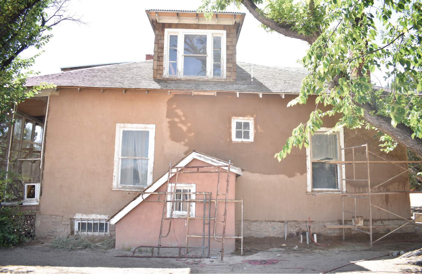
Mud plastering in progress at the Pino House, Las Golondrinas, photo by Ramon Dorado
