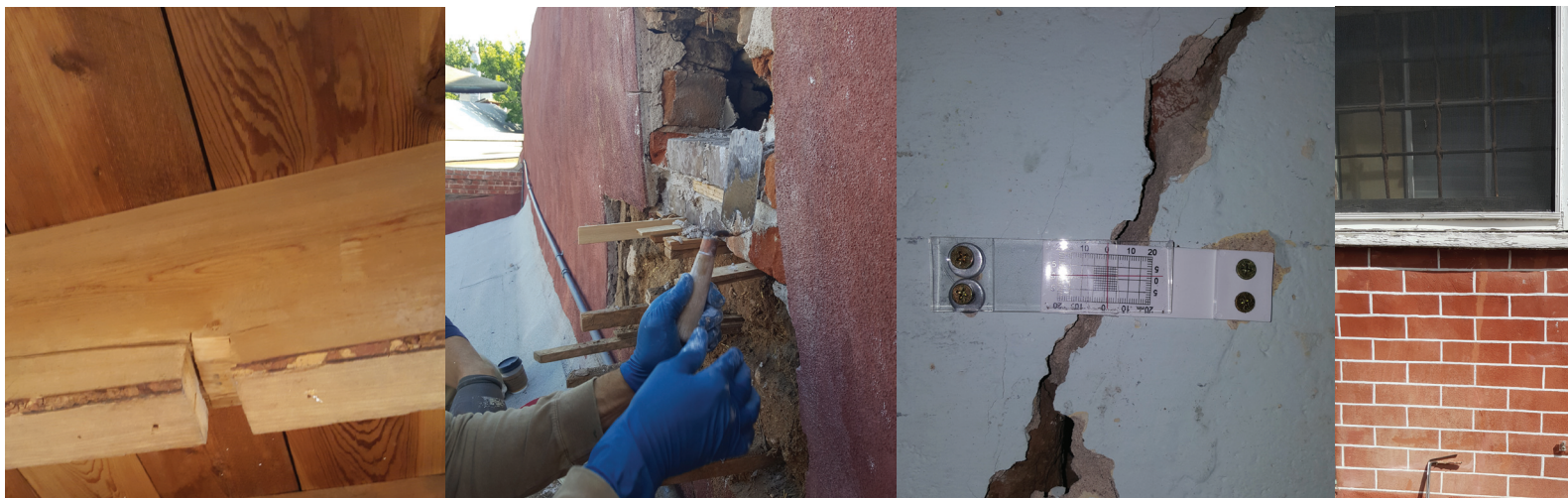
Left to right: Ceiling beam in need of repair; parapet repair in progress; crack monitor inside building; plaster crack on outside of Hovey House; Mac Watson explains how to probe a
