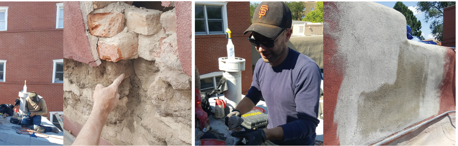
mortar sets; Jay Dickason removing damaged parapet bricks; damaged adobe and fired bricks prior to parapet repair; Jay Dickason applying lime mortar; Freshly finished parapet repair
