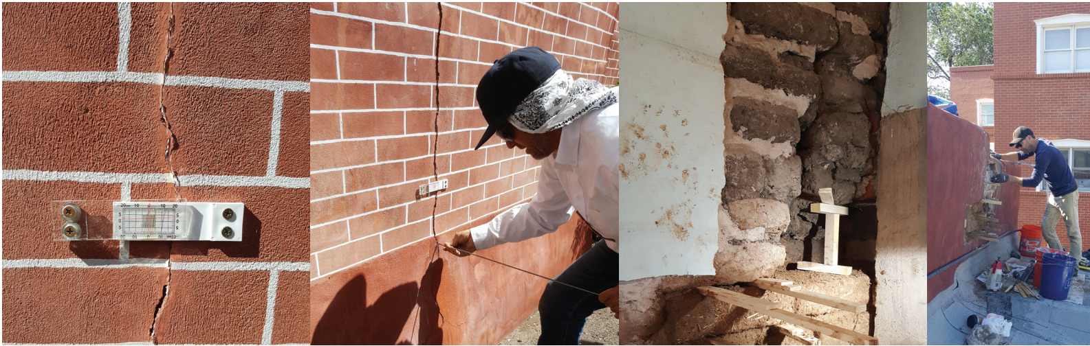
Left to right: Crack monitor on outside of Hovey House; Bobby Wilson probing a crack to find out the extent of damage; adobe repair in process with new adobes shimmed as their
